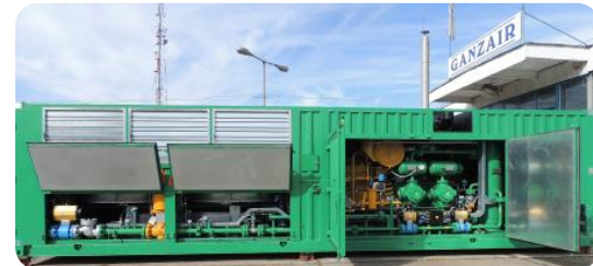
Evacuation Compressor Units
