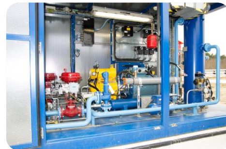
Flare Gas Compressor
